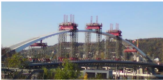
Use of the PIZMO structure for the lifting of a permanent bridge construction
